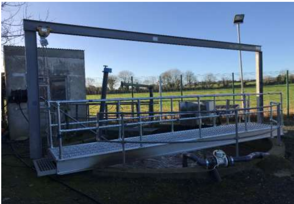
Gantry & Lifting System at Tinryland WWTP
